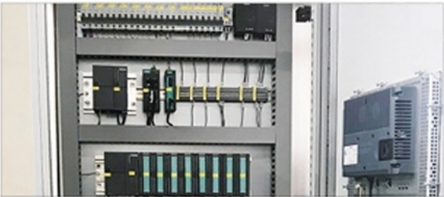
PLC 柜内 Inside the PLC cabinet
